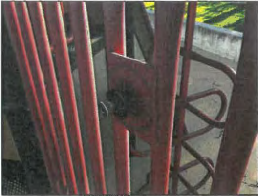
7. Protrusion and missing equipment
