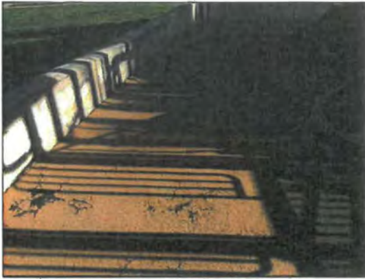
19. Damaged poured in place surfacing
