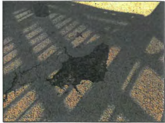
20. Damaged poured in place surfacing
