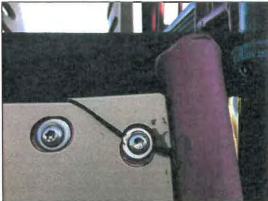
3. Cracked rock climbing wall
