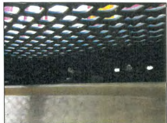
6. Protrusions on bolts underneath platform
