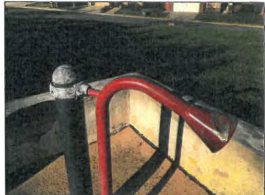
4. Corroded and damaged fun fone
