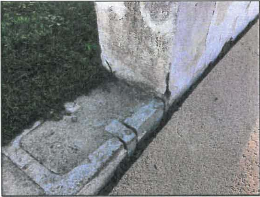
13. Trip hazard at east end of play area
