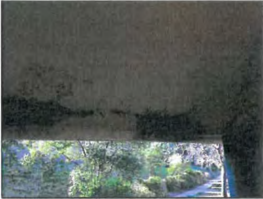
1. Mold underneath roof
