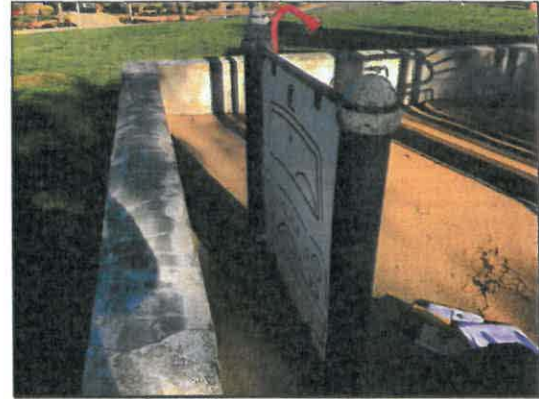
16. Play panel too close to concrete wall
