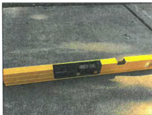
23. Grade exceeds 2% on access walk
