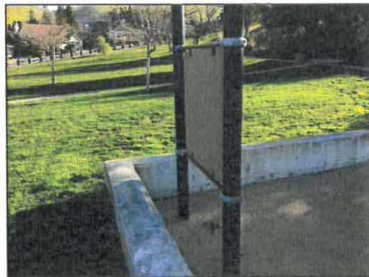
17. Play panel too close to concrete wall
